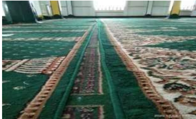
Figure 3. The Condition of the Floor of the Main Room of the Mosque
