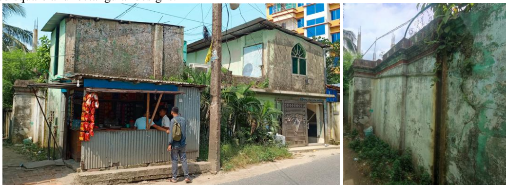
Fig.18 Present Condition of Yousufganj Mosque,It's Effects, Building Materials. Photos by, Author.
