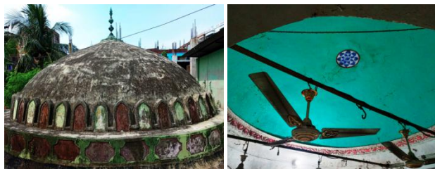
Fig.11 Exterior and Interior View of Yusufganj Mosque Dome, Photography by, 1 st Author
