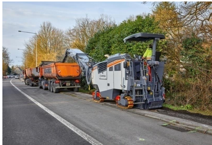
Figure : Milling machine removes asphalt pavement layers as part of pavement rehabilitation.
