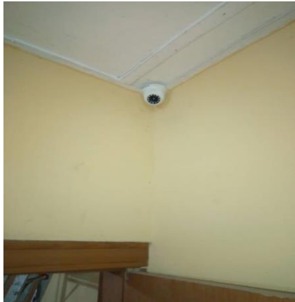
Figure 5: Installed Camera at the Deputy Rector's Office Walkway
