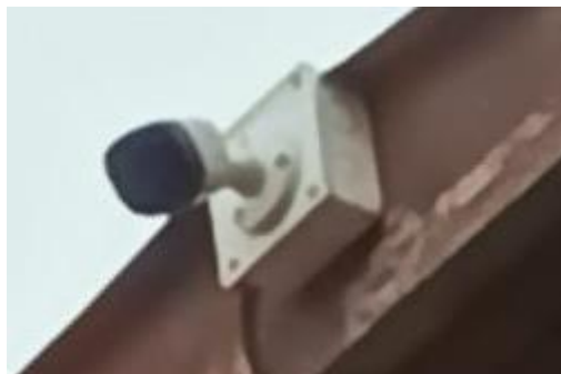
Figure 4: Installed Camera at the Deputy Rector's Office.
