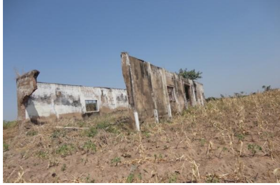
Figure 2. Dilapidated warehouse at Korinya service centre
