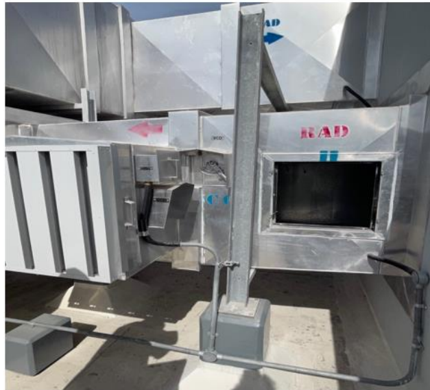
Fig 3.2: Return Air Sensor Near Fresh Air Intake
