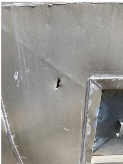
Fig 3.1: Air Leakage In Duct
